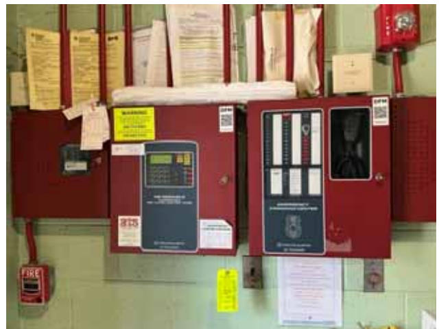
24 - FIRE ALARM PANEL
